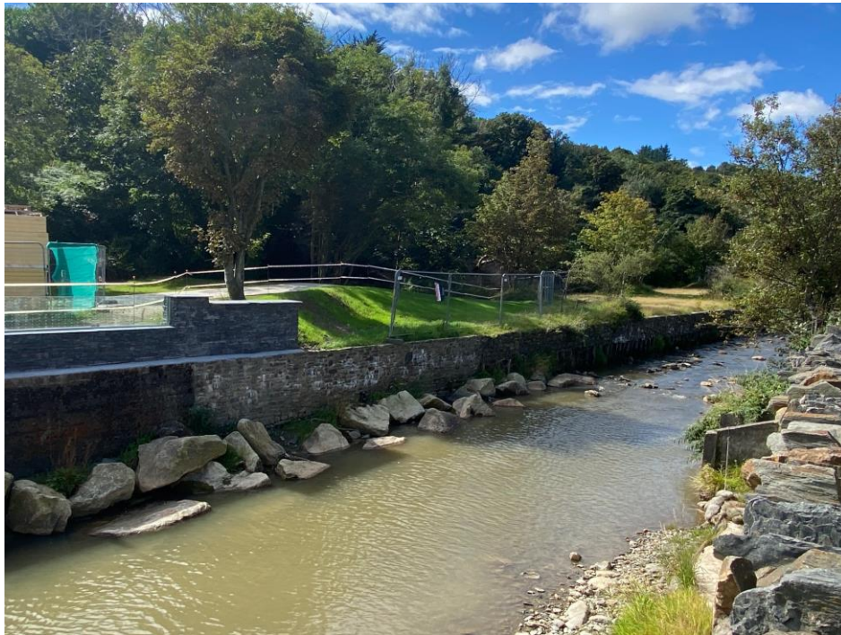
Above shows the newly created bund and ramp. Also shown is part of the new river defence wall.
