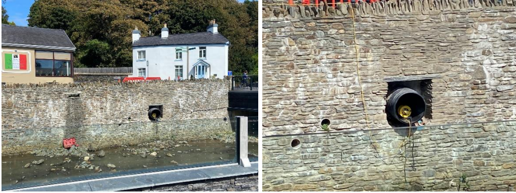
The 60cm diameter surface water drain outlet is shown above, this water pipe takes the surface water from road side gullies and links in to the pipe collecting water from Lower Cronk Orry
